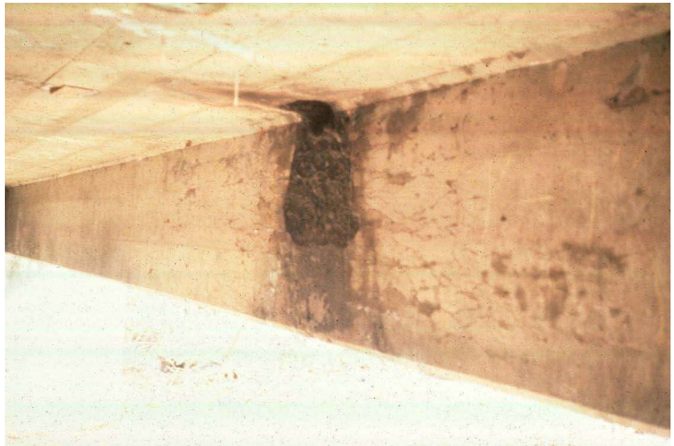
Figure 9.2.18 Deteriorated Tee Beam Stem Adjacent to Drain Hole
