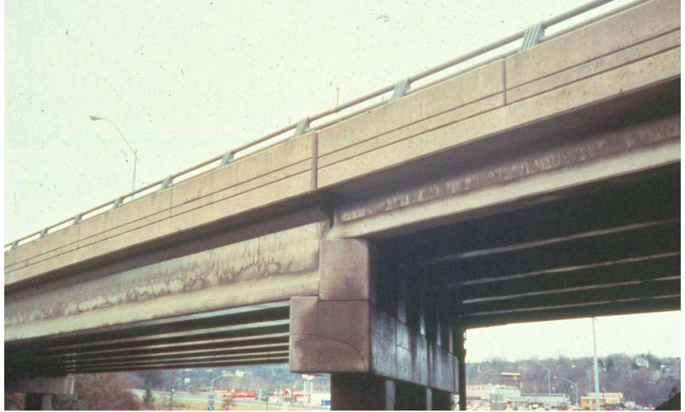
Figure 9.9.19 Leakage of Water at Joint between Spans
