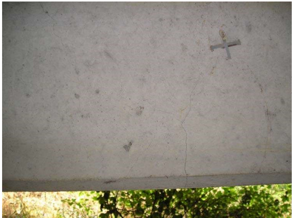
Figure 9.2.13 Flexure Cracks on a Tee Beam Stem
