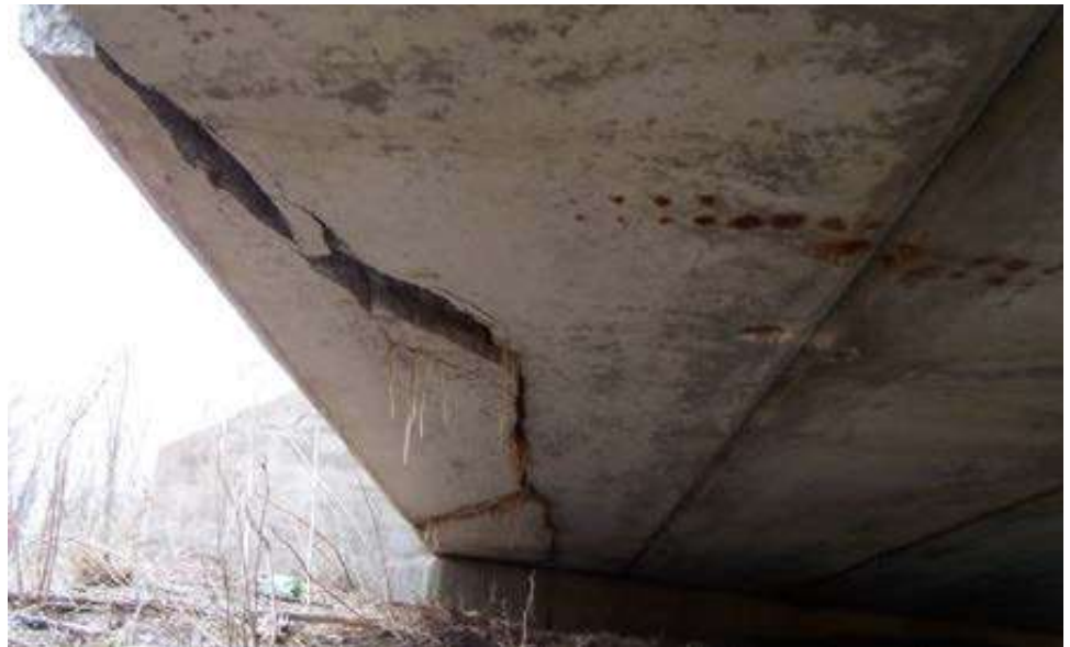
Figure 9.10.18 Close-up of Box Beam Collision Damage
