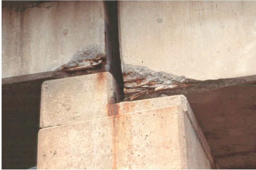
Figure 9.10.11 Spalled Beam Ends with Exposed Prestressing Reinforcement
