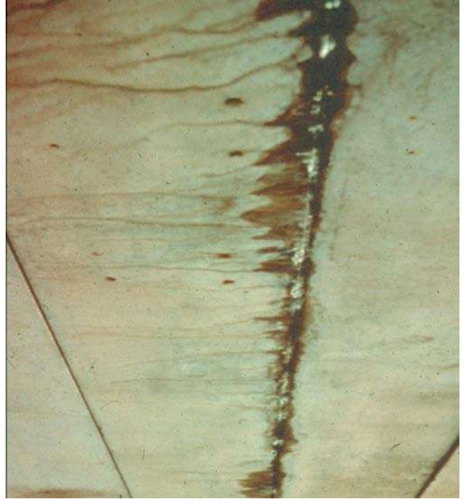
Figure 9.7.6 Leaking Joint between Adjacent Slab Units
