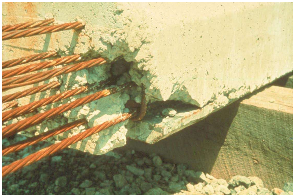
Figure 9.9.16 Spalling Due to Poor Concrete Placement
