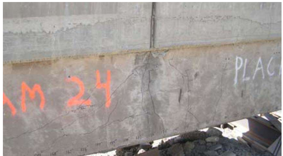
Figure 9.10.28 Cracking Near Barrier Joints
