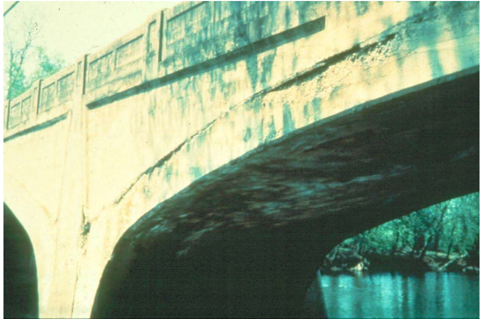
Figure 9.5.15 Deteriorated Arch/Spandrel Wall Interface
