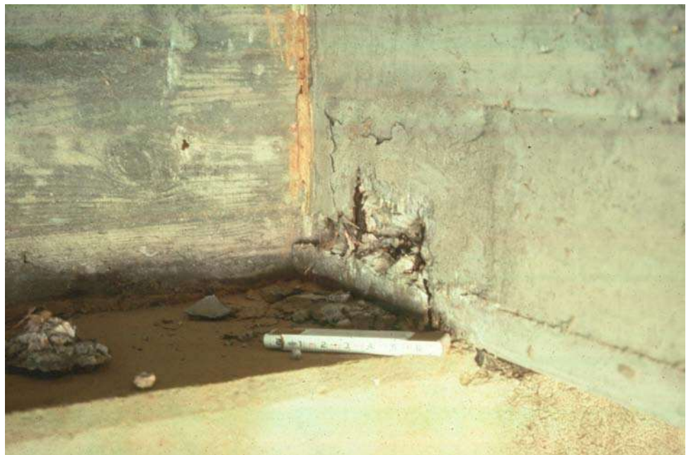
Figure 9.2.10 Deteriorated Tee Beam Bearing Area
