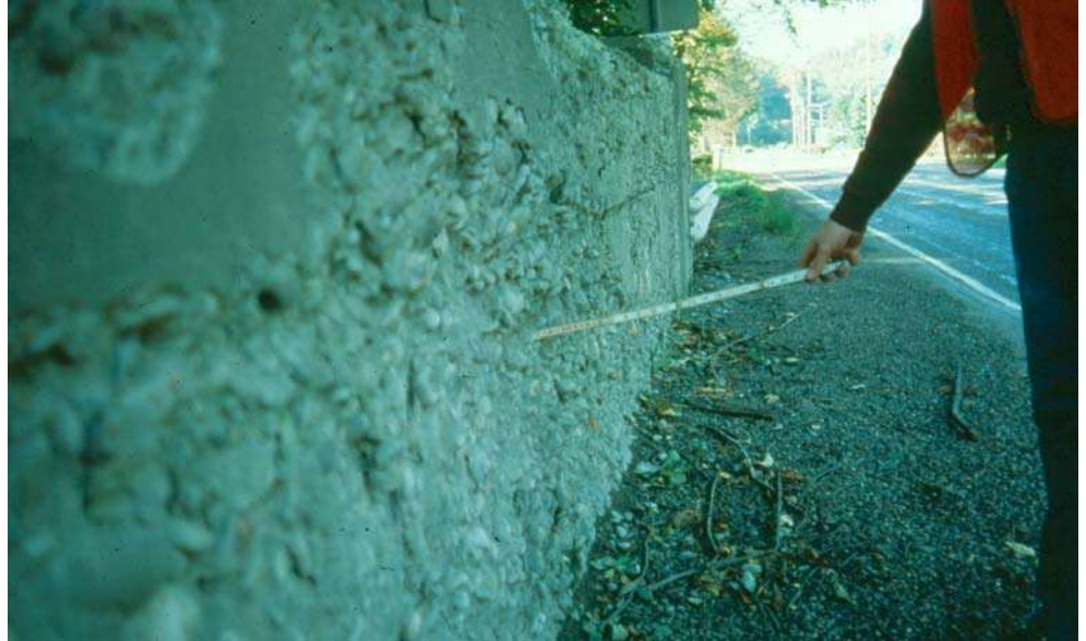
Figure 9.3.9 Close-up of an Interior Face of a Through Two-Girder with Heavy Scaling due to Deicing Agents
