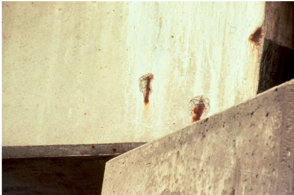
Figure 9.10.12 Exposed Shear Reinforcement at End of Box Beam
