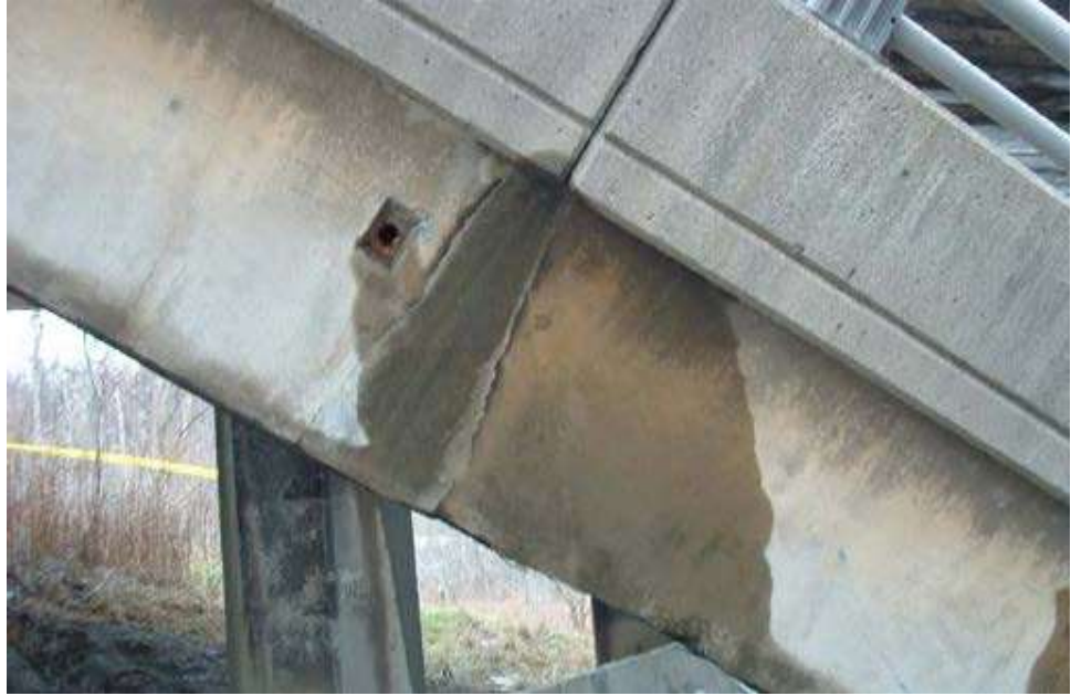
Figure 9.10. 29 Water Leakage Through Parapet Deflection Joints
