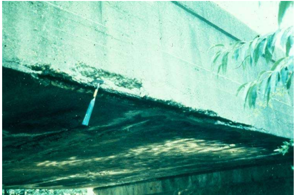
Figure 9.3.8 Exposed Reinforcement in a Through Two-Girder (under hammer)
