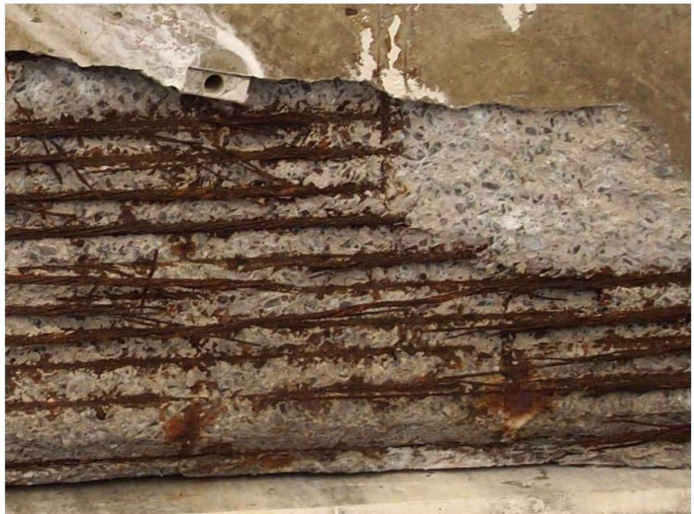
Figure 9.10.16 Close-up of Failed Strands due to Corrosion
