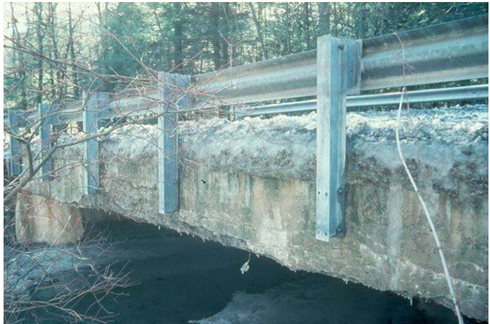
Figure 9.1.9 Deteriorated Slab Fascia due to Roadway Deicing Agents
