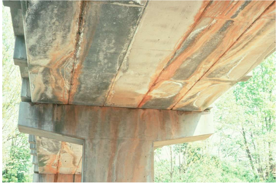
Figure 9.10.17 Joint Leakage and Rust Stain
