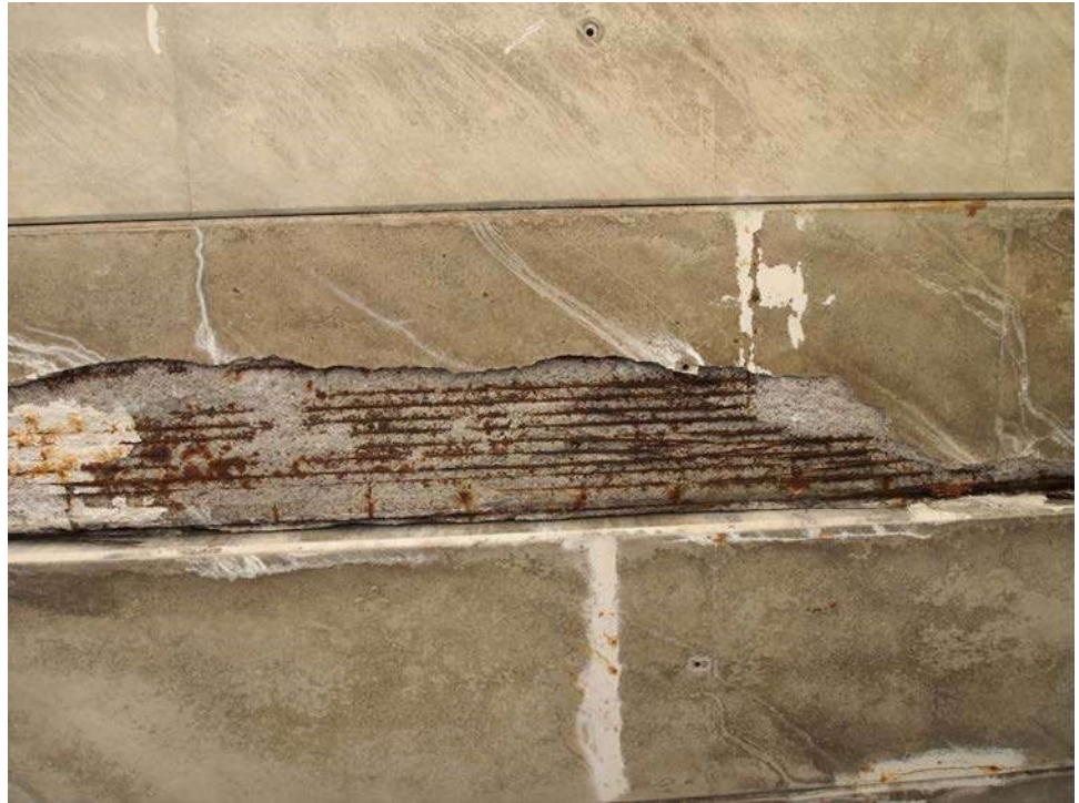
Figure 9.10.15 Spall and Exposed/Corroded Reinforcement
