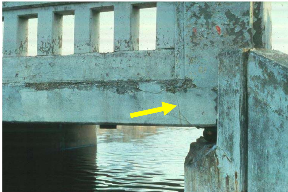
Figure 9.1.5 Diagonal Shear Cracks Close to the Ends of a Slab Bridge
