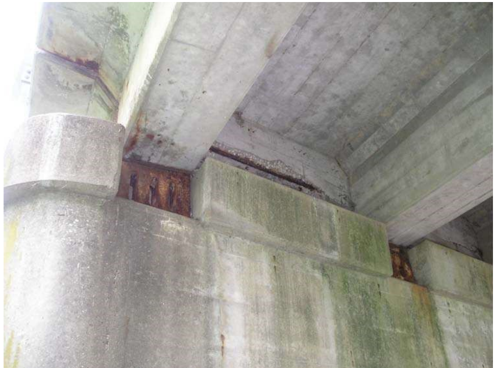
Figure 9.2.12 Shear Zone of Cast-in-Place Concrete Tee Beam Bridge
