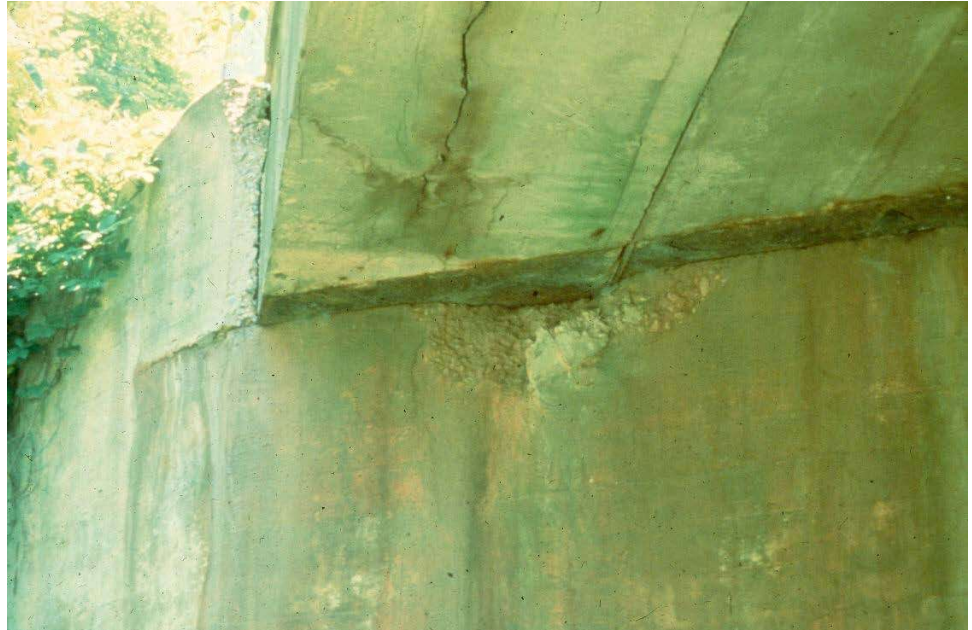
Figure 9.10.13 Longitudinal Cracks in Bottom Flange of Beam
