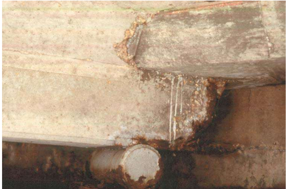
Figure 9.2.9 Spalled Tee Beam End
