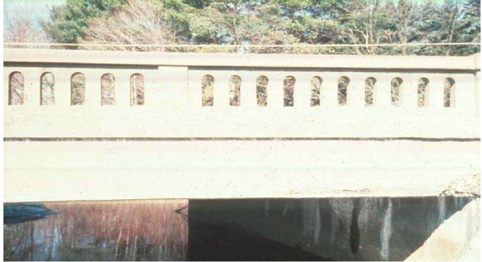
Figure 9.2.19 Deteriorated Tee Beam End Due to Drainage
