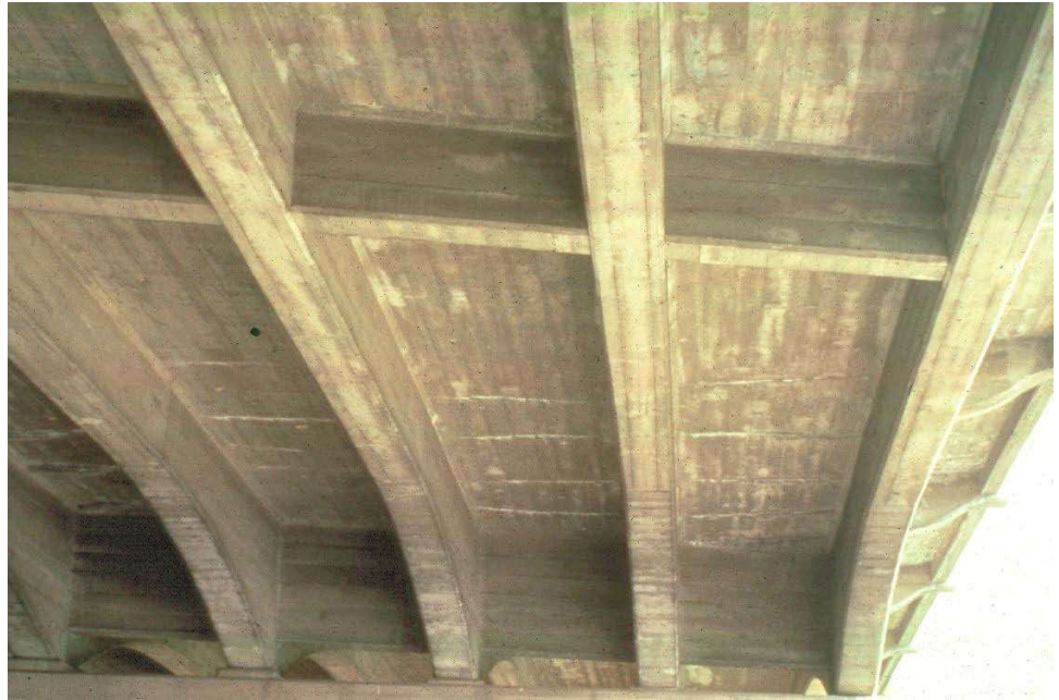
Figure 9.2.14 Flexure Cracks in Tee Beam Flange/Deck
