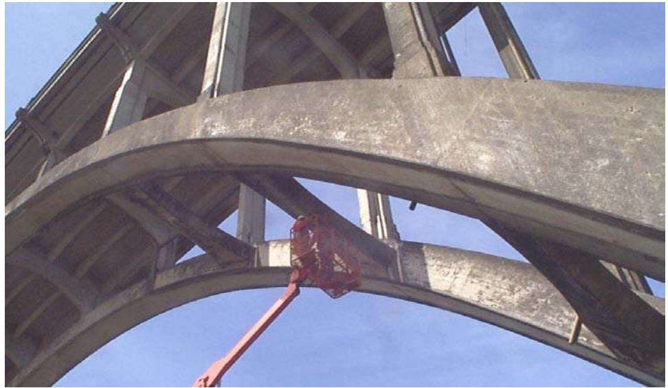
Figure 9.5.17 Inspection and Documentation of Arch Strut Deficiencies
