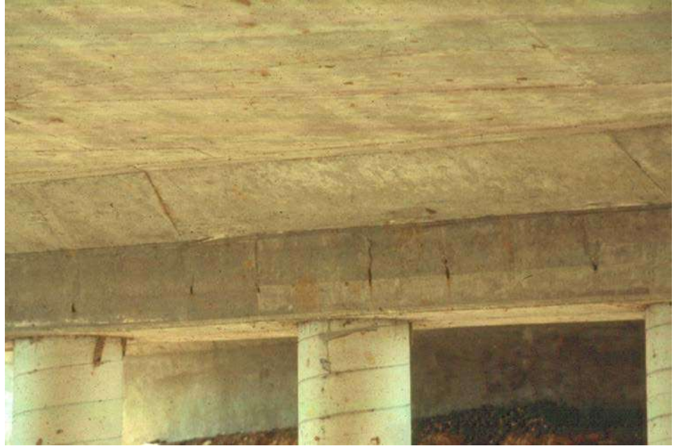
Figure 9.1.6 Shear Zone on the Underside of a Continuous Slab Bridge Near a Pier
