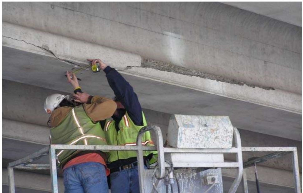
Figure 9.9.20 Inspectors Evaluating Collision Damage on Prestressed Concrete I-beam
