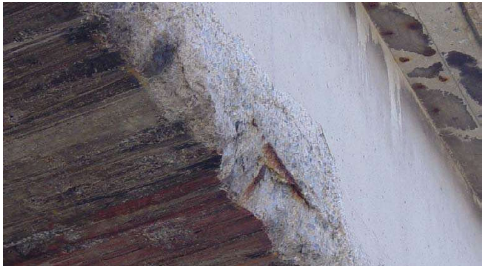
Figure 9.2.20 Collision Damage to Tee Beam Bridge Over a Highway
