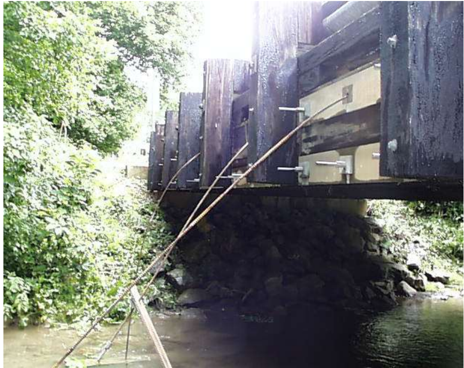
Figure 8.3.10 Broken Stressing Rods
