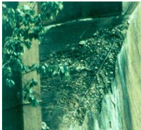
Figure 9.5.18 Scaling and Contamination on an Arch Rib Due to a Failed Drainage System
